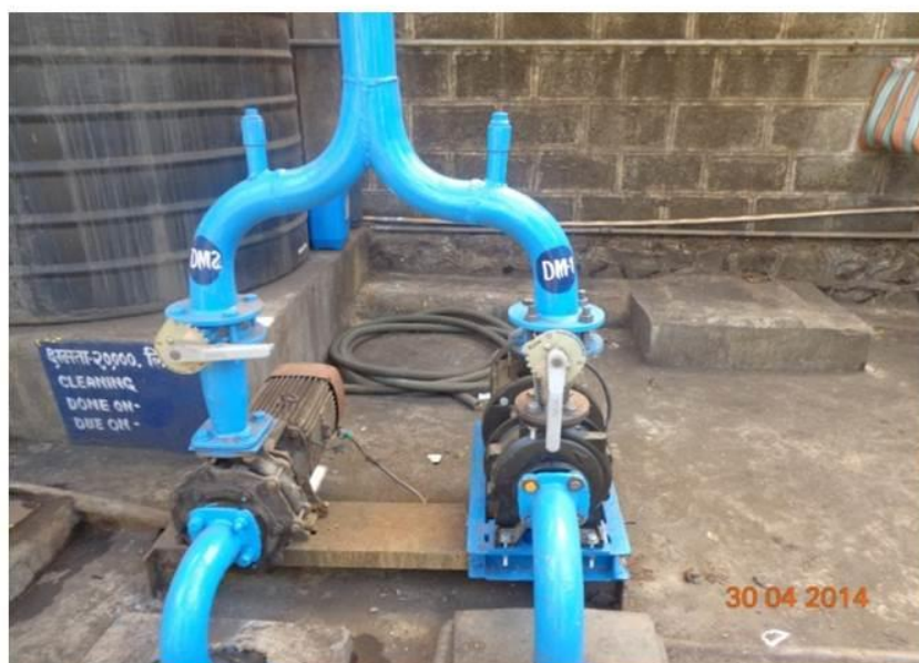
Proper sizing of pump and improving energy efficiency
